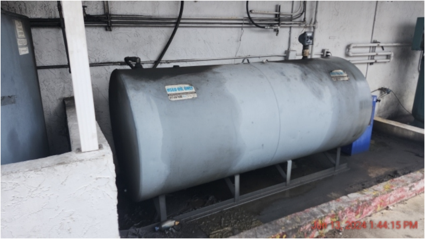
Photo 15: 500-gallon waste oil above ground tank in bermed roofed area outside the Central Main Shop.
