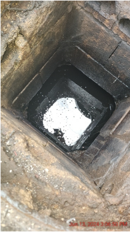
Photo 46: Inside view of oil-water separator located adjacent to the old dodge shop
