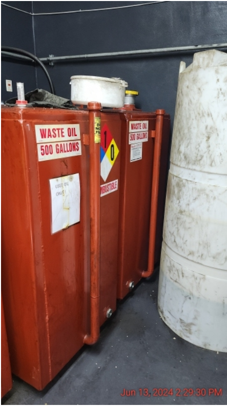
Photo 36: Close-up of the 500-gallon used oil above ground tank.
