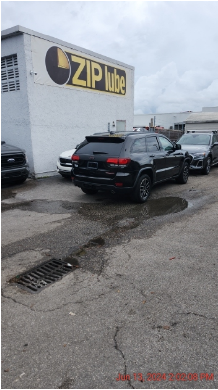
Photo 25: overview of southern storm drain located near the quick lube shop next to the manual car wash
