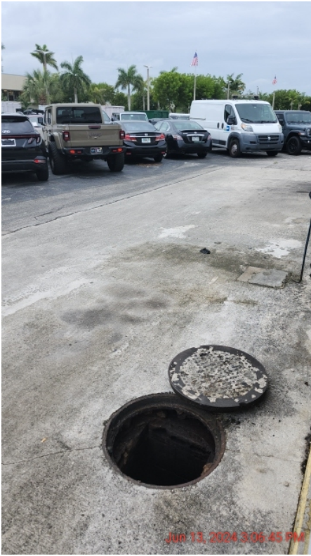
Photo 45: Overview of oil-water separator located adjacent to the old dodge shop
