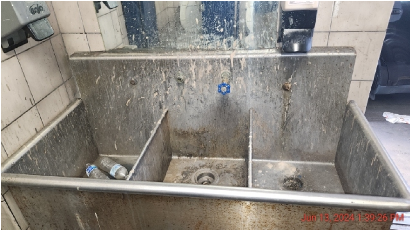
Photo 12: hand sink located in the restroom area
