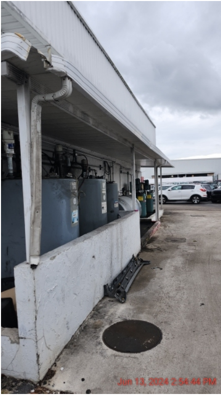
Photo 43: Overview of oil-water separator located in between the central maintenance shop and the quick lube station
