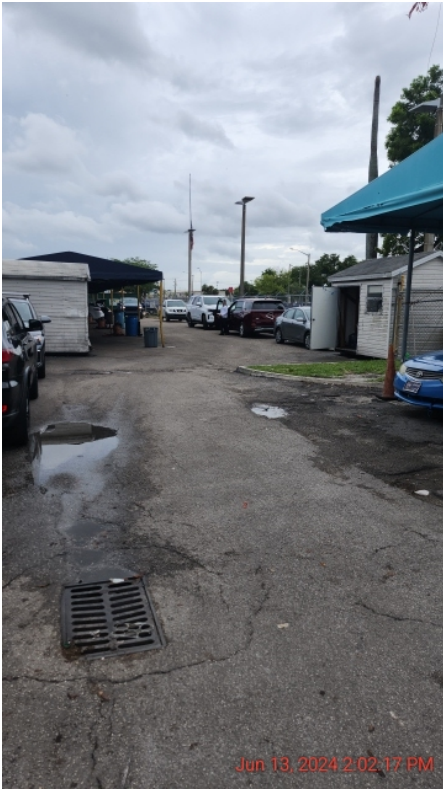
Photo 26: overview of southern storm drain located near the quick lube shop next to the manual car wash (continued)
