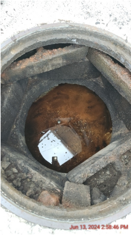
Photo 44: inside view of oil-water separator located in between the central maintenance shop and the quick lube station
