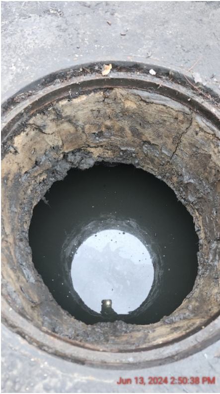
Photo 42: inside view of oil-water separator located near car wash
