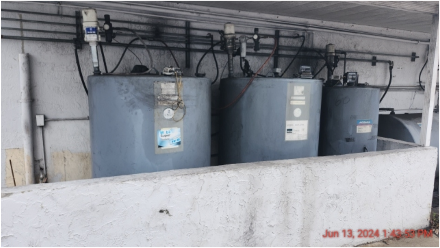
Photo 14: three 250-gallon above ground tanks of fresh oils in bermed roofed area outside the Central Main Shop.
