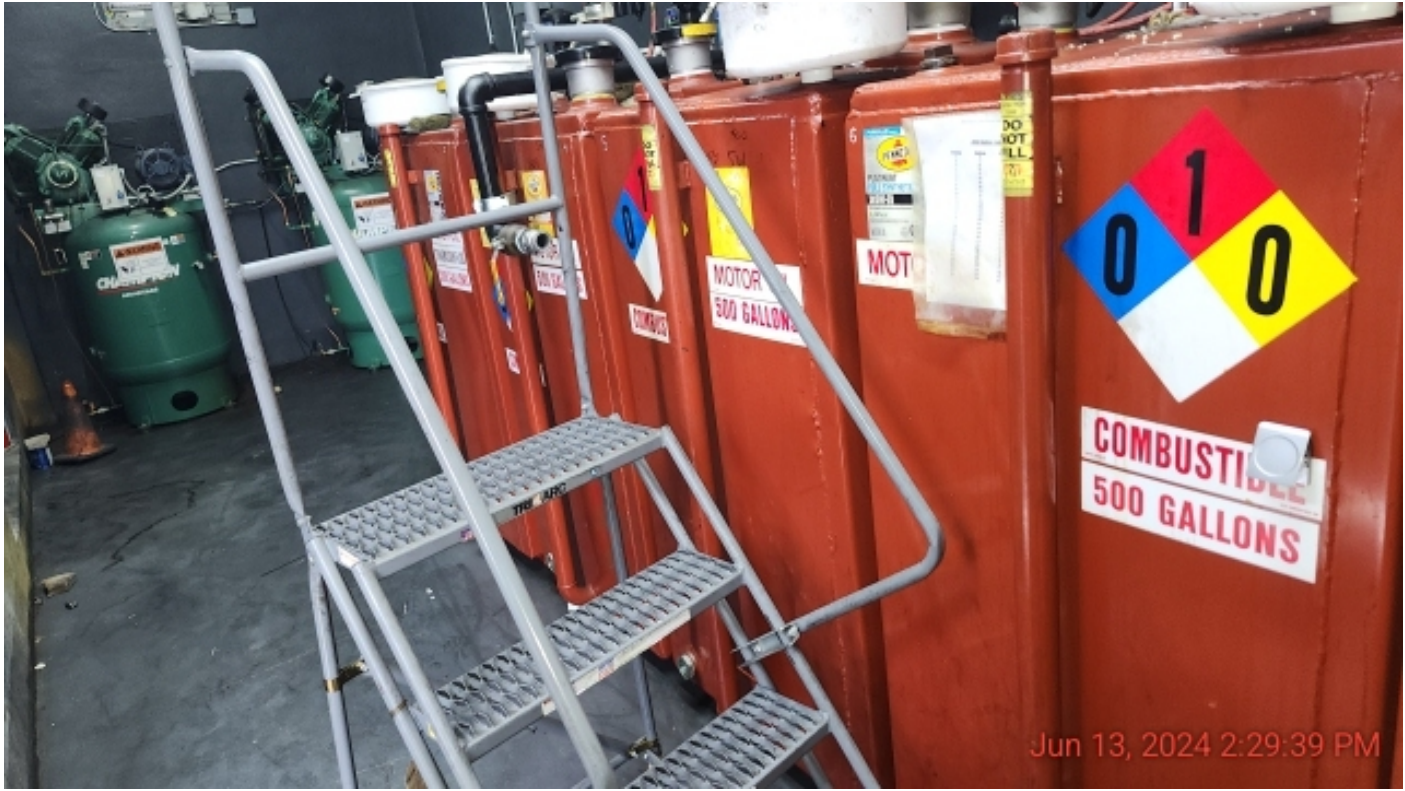
Photo 37: Overview of the new oils in the above ground tank storage room.
