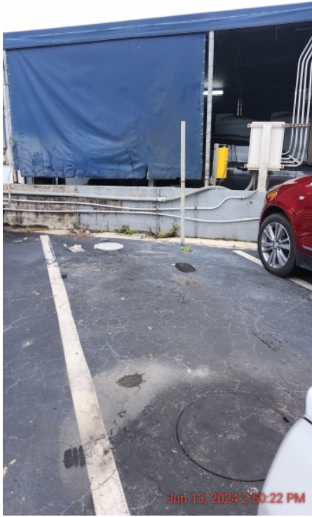
Photo 41: Overview of oil-water separator located near car wash
